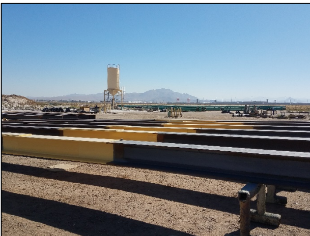
Figure 5: In total, Mobile Pipe coated 51 H-piles for the new Shelter Island Boat Launch facility.
