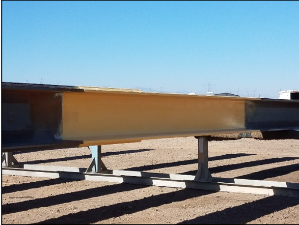
Figure 3: 80mils of Polibrid® 705E applied in 10-foot sections for corrosion protection of each H-pile. Polyurethanes offer great corrosion protection in salt water environments and are tough enough to handle the piling application.
